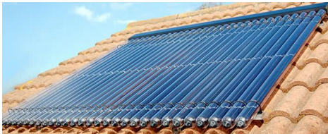
Solar Heating Panel
