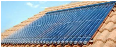
Solar Heating Panel
